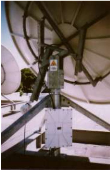
Figure 9: View of terminals on the roof of University of Hawaii building, showing white cast box containing microwave electronics
