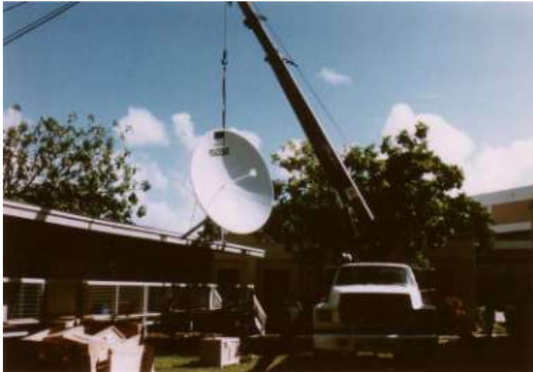
Figure 10: Terminal being lifted on to the roof of University of Hawaii building during installation by MAS
