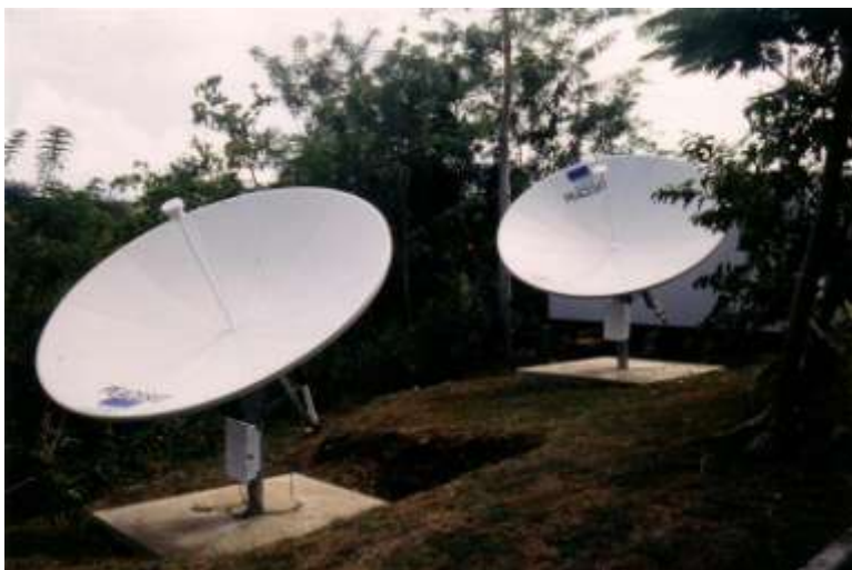
Figure 6: Terminals installed at the Forum Fisheries agency in Honiara, Solomon Is, showing concrete mounting pedestal.
